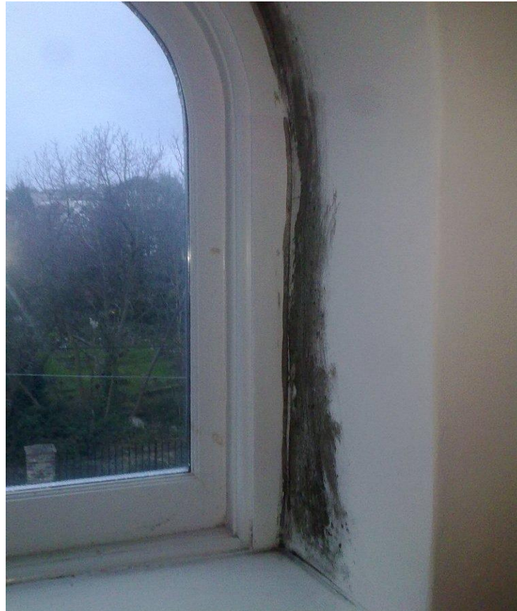
At the surface
